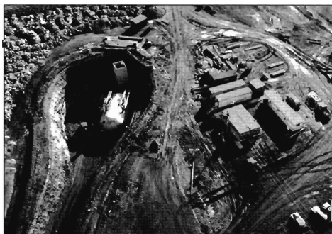
The U.S. Army Corps of Engineers built South Dakota's 15 underground Minuteman missile launch control centers in the early 1960s.
